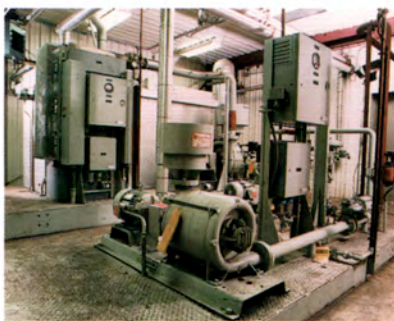
Twenty foot long metal sheath thermocouple probes monitor injection temperatures in this flue gas conditioning system.
