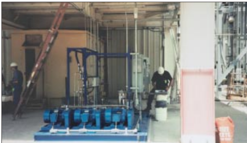
Braden Fogging System located at a Texas gulf coast chemical company sized for a frame 7EA gas turbine
