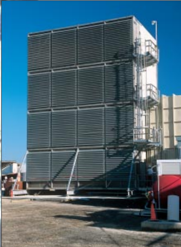
Barrier filter with evaporative cooler for a Westinghouse 501F in Texas, USA.
